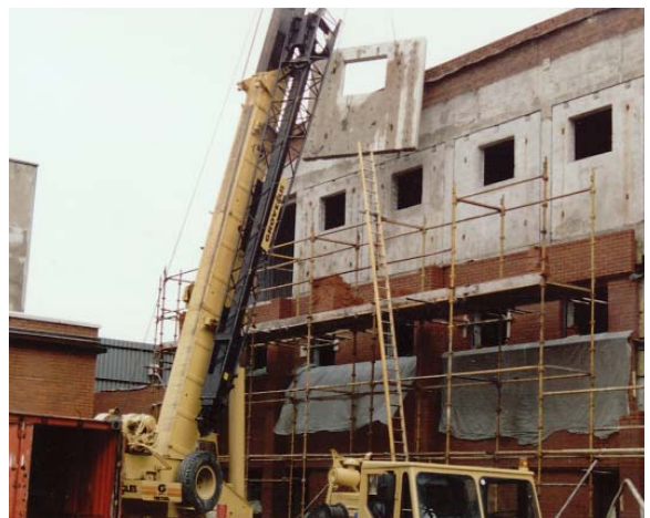
MODULAR Precast concrete panel assembly sped construction pace, and minimized risk to work force.
